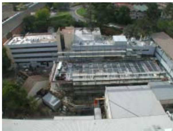
Stages in the construction of the new wing of the Cockcroft Building as captured by the automated skycam: top, the old Round House. middle, the cleared site. bottom, the new wing under construction
